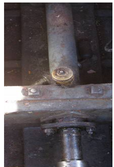
Figure 4-9: Propeller Shaft Bearing
