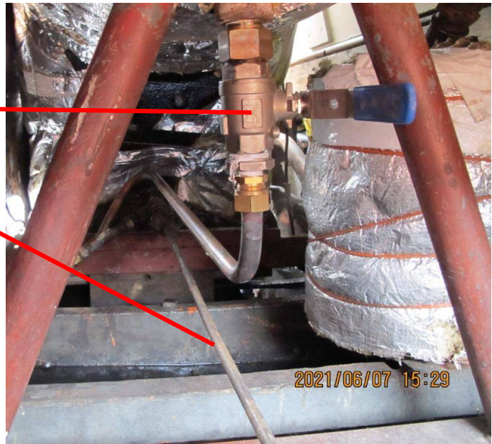
Figure 7-1: Blow down valves (photo taken before the boiler casing was fitted)
