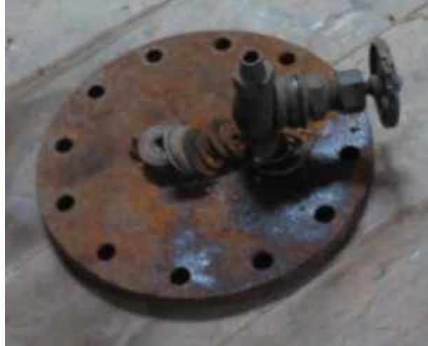
Figure C-5: Steam Dome Blanking Flange
